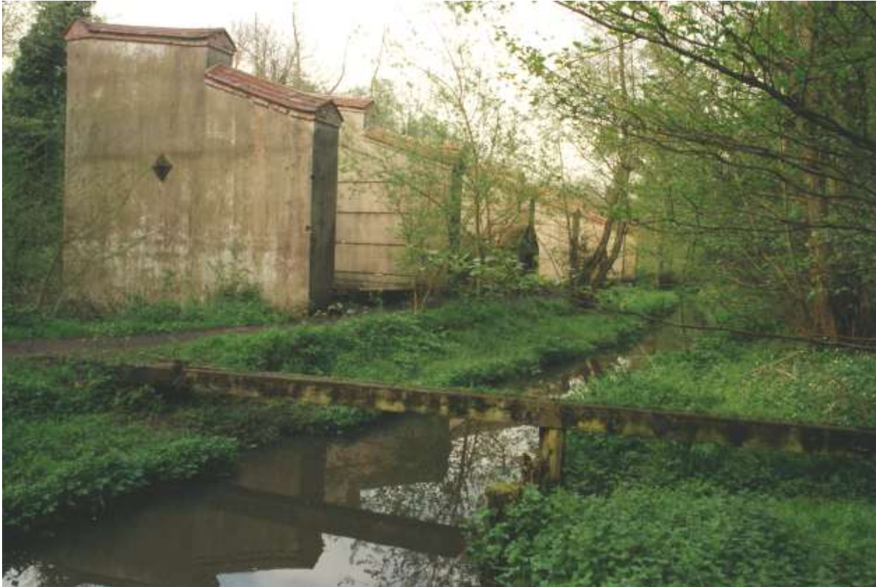
Remains of a range of steam-powered gunpowder incorporating mills at Chilworth, built in 1885.
